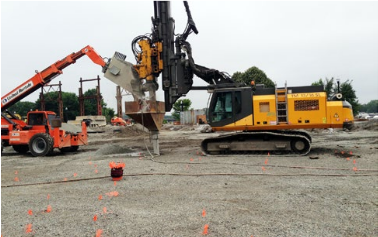
▶ A Geopier® Rammed Aggregate Pier® crew operates on a well-prepared Working Platform
