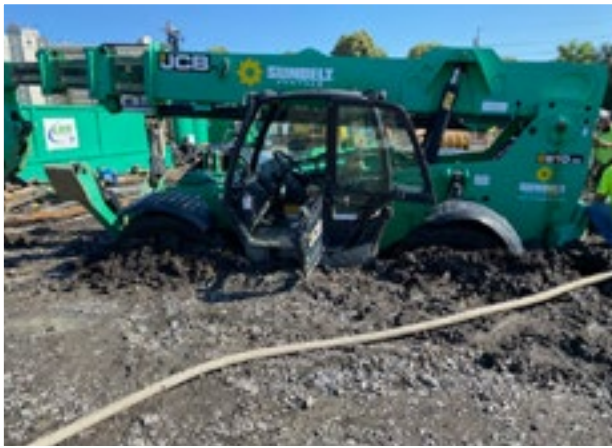
► A lull for concrete formwork is stuck after attempting to traverse an unstable Working Platform.
