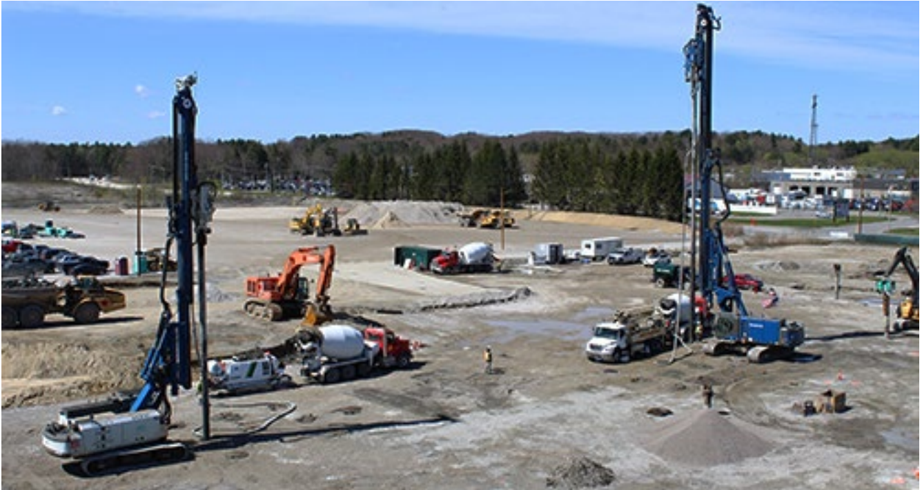
► Two Geopier® GeoConcrete® Column (GCC) rigid inclusion crews operate on a well-prepared Working Platform.
