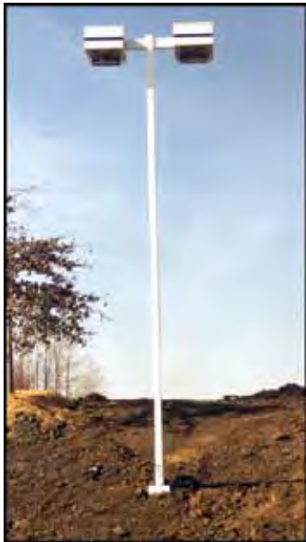
Installed Light Standard Figure 10-2
